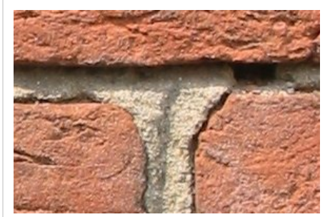
Mortar holding weathered bricks
