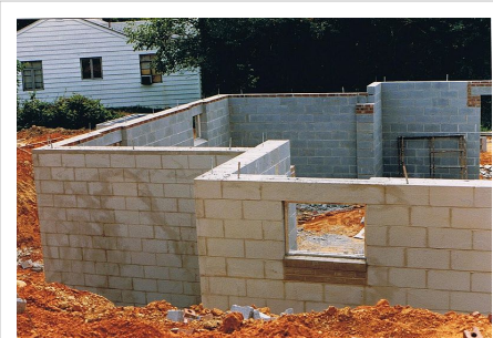
Concrete masonry units (CMUs) or blocks in a basement wall before burial.
