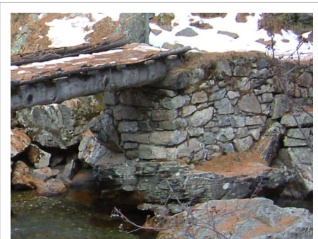
Dry set masonry supports a rustic log bridge, where it provides a well-drained support for the log (this will increase its service life).
